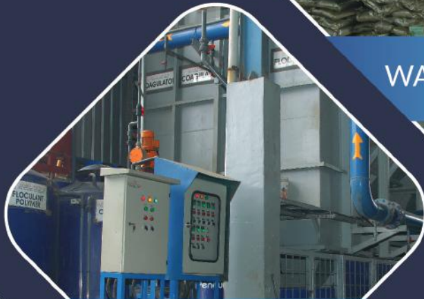
WASTE WATER TREATMENT
